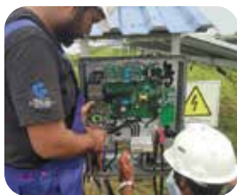
Inverter Services (Solar)
